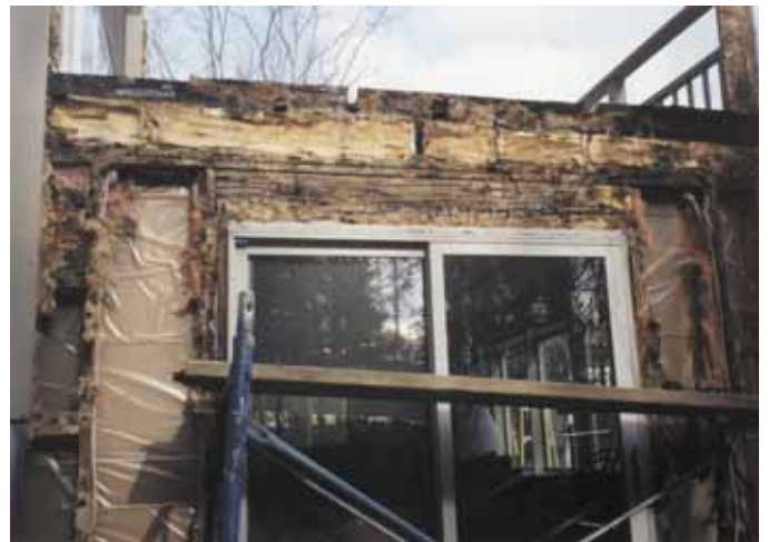
Photograph 5: Failure on Steroids —Note the plastic vapor barrier “accelerant” in this Vancouver, Canada building.
