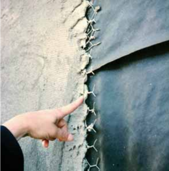
Photograph 2: Hardcoat Stucco —Three coats have been traditionally applied directly over a single layer of impregnated felt or asphalt saturated kraft paper. Today, this results in a bond between the stucco rendering and the outer layer of the felt or paper compromising drainage.
