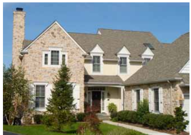
Photograph 1: Pennsylvania Stucco “Shack” —Eastern Pennsylvania is the stucco failure capital of the United States. Note the manufactured stone veneer—or “lumpy” stucco on the front façade.
