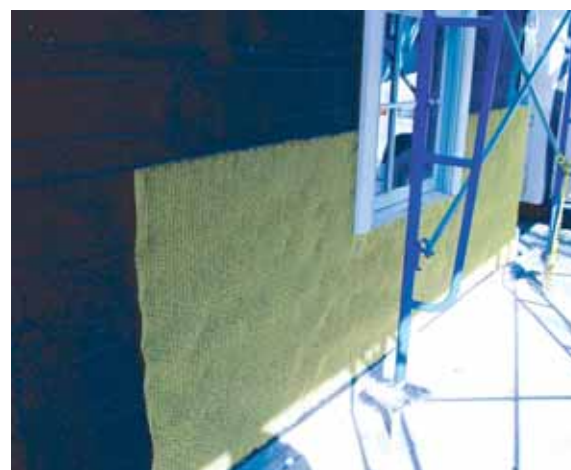
Photograph 8: Air Gap —The air gap does not have to be particularly big to be a big deal—3/8 inch (9 mm). One method of getting the air gap is to use a drainage mat between two layers of building paper. The gap allows redistribution of the moisture in both the stucco and the OSB sheathing.
